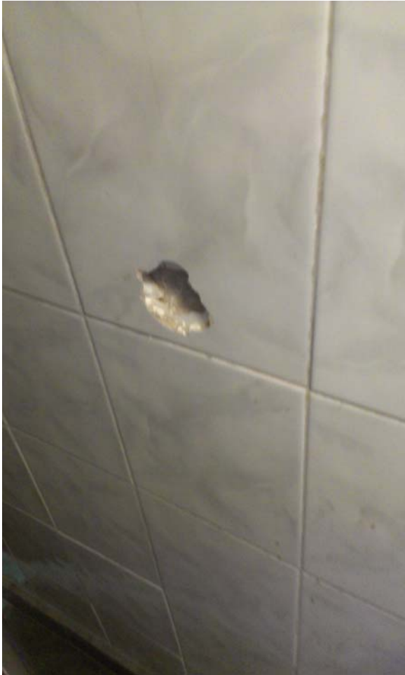
6) Damaged tiles left unrepaired.
