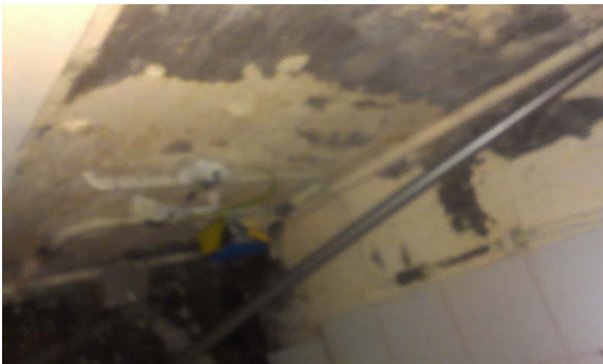
17) Very poorly maintained toilet facilities.
