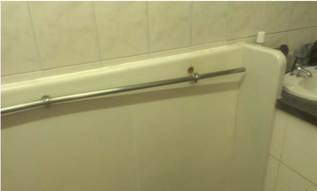
2) Damaged water pipework in toilet area.
