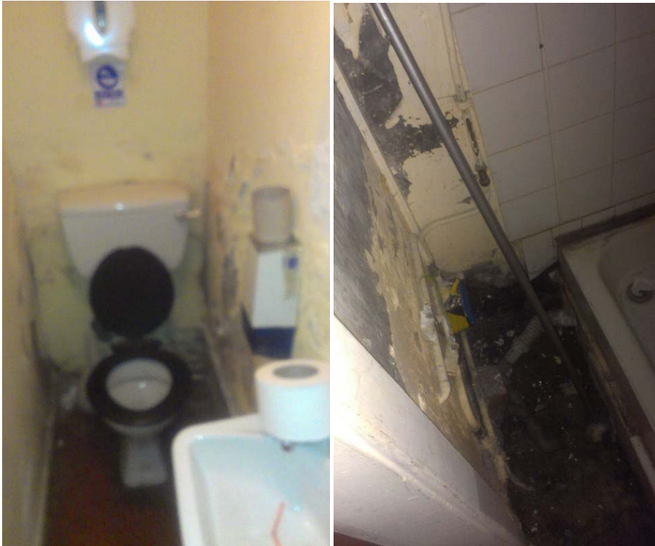
16) Very poorly maintained toilet facilities.
