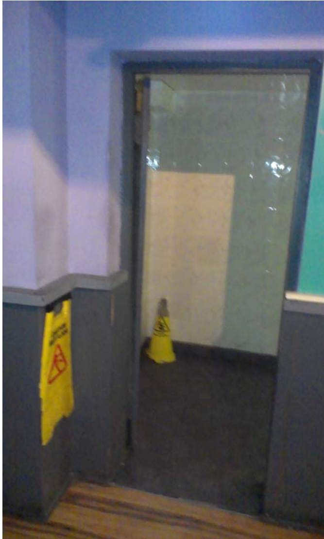
12) Wet floor signs in permanent use.
