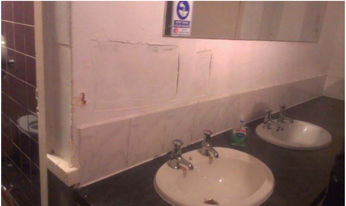
11) Poorly maintained wash facilities.
