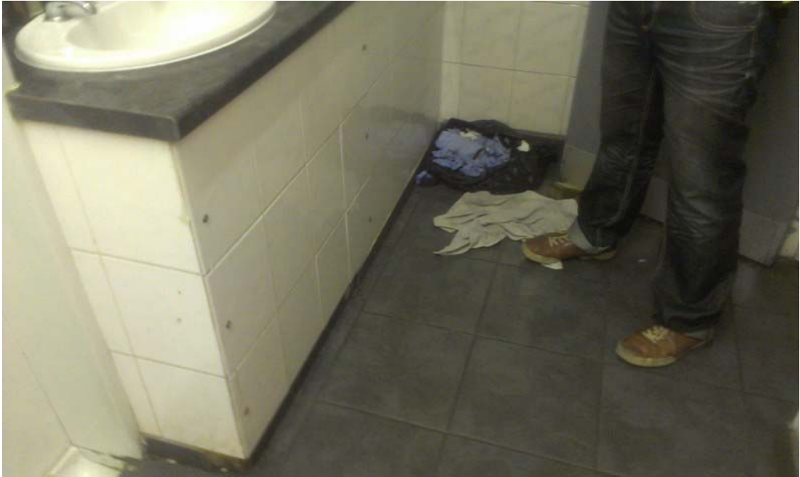
3) Poorly maintained toilet facilities-waste on floor.
