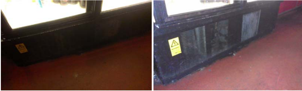
3) Poor cleanliness of cooler ventilation.
