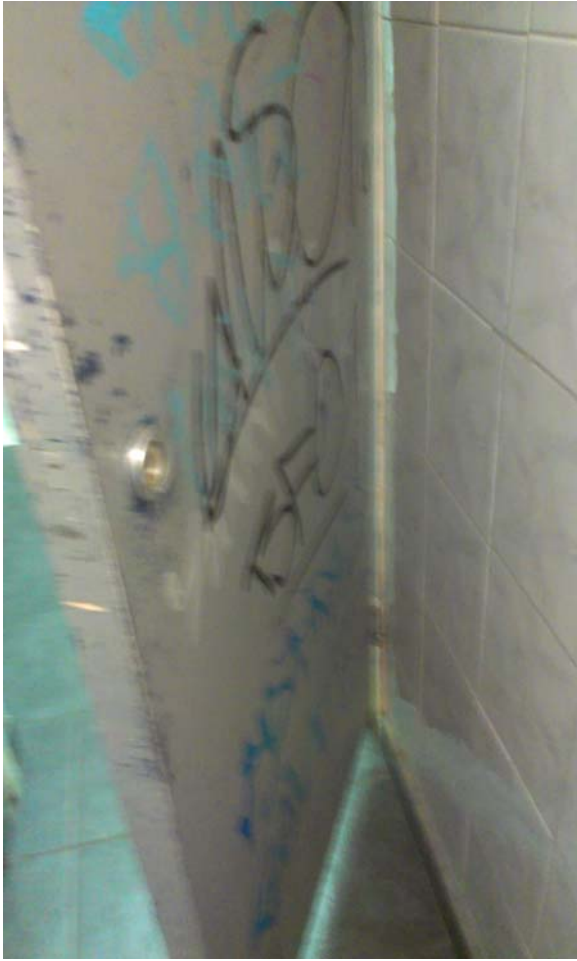
7) Locks missing from toilet doors.
