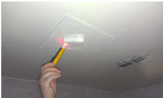
11) Temporay repair with tape not IPX rated.
