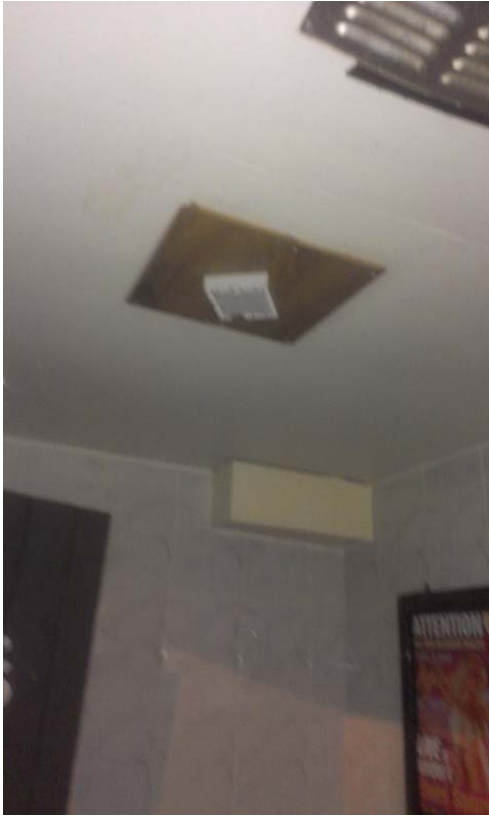
7) Damaged electrical furniture comprising IPX ratings.
